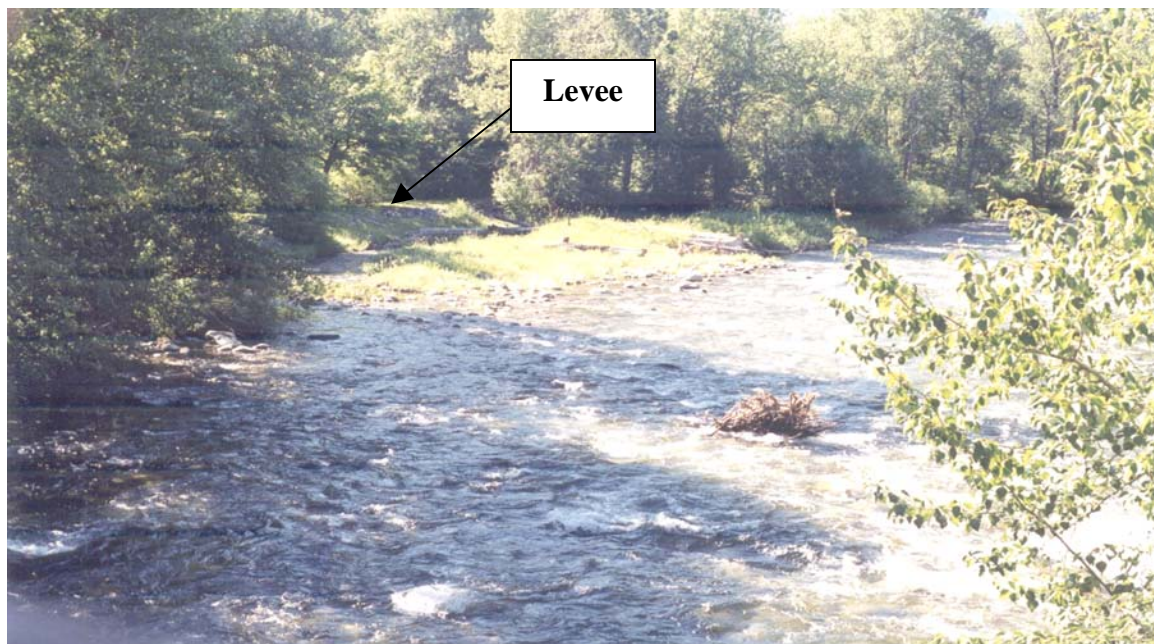
Figure 24. Present-day view of an old levee feature located downstream of the Roaring Creek Bridge. Most of the levee and bank protection features are difficult to discern from the landscape because of their inconspicuous size and the fact that many are now covered by dense vegetation.
