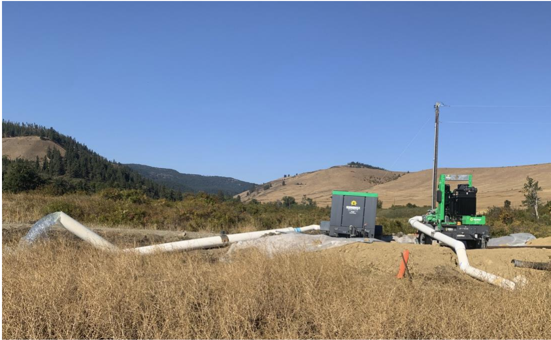
Figure 1. Pump and discharge point configuration.
